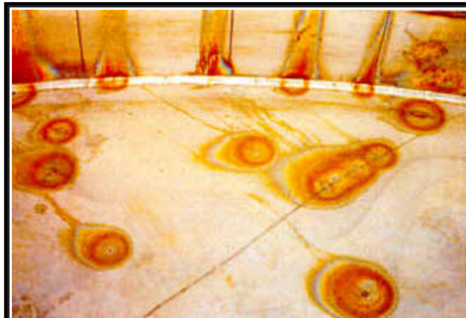
Fig 3: Corrosion effects on the bottom
